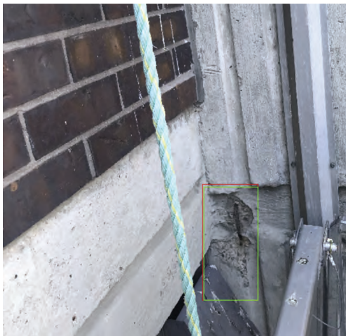
Fig. 4: Double positive indication—spall and exposed rebar
