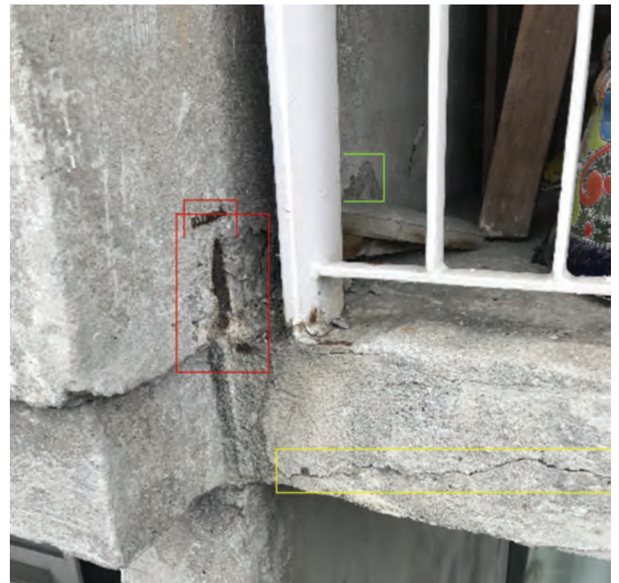
Fig. 5: Example of AI condition detection (red boxes display detected exposed rebar, green—spall, yellow—crack)
