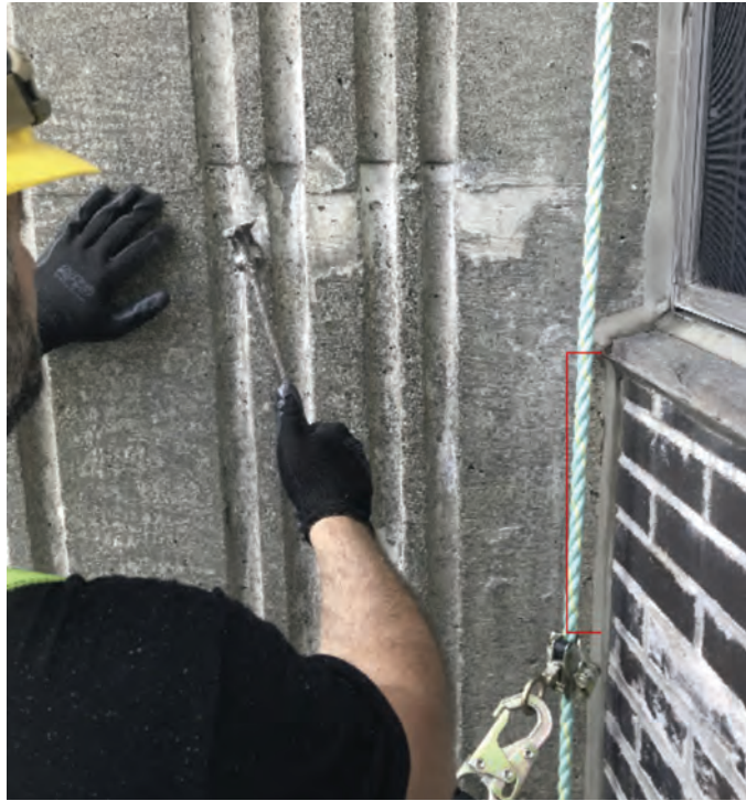
Fig. 3: False positive indication—lifeline detected as exposed rebar
